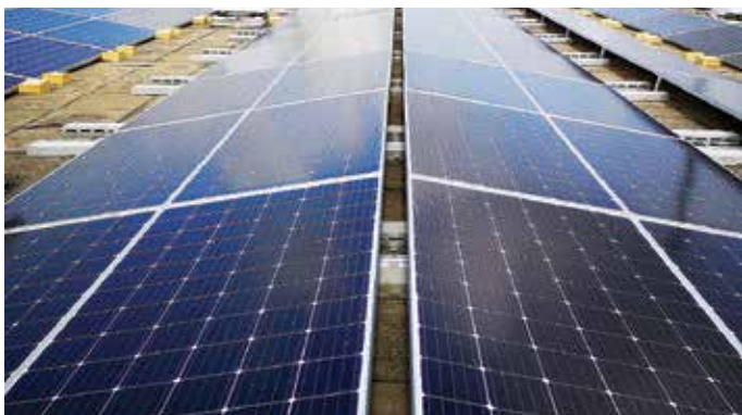
YTL PowerSeraya completed the installation of 970.5 kWp solar project in February 2019
