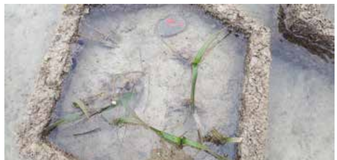
Seagrass contained in hexagonal hollow concrete blocks to minimise soil loss caused by strong currents and wave attrition
