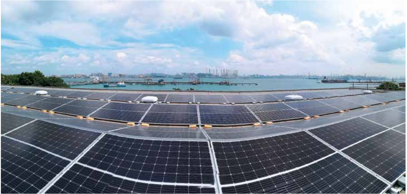
⚡ Part of the solar PV installation at YTL PowerSeraya power plant in Jurong Island, Singapore
