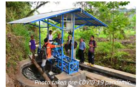
Micro hydro unit installed by YTL Jawa Timur
