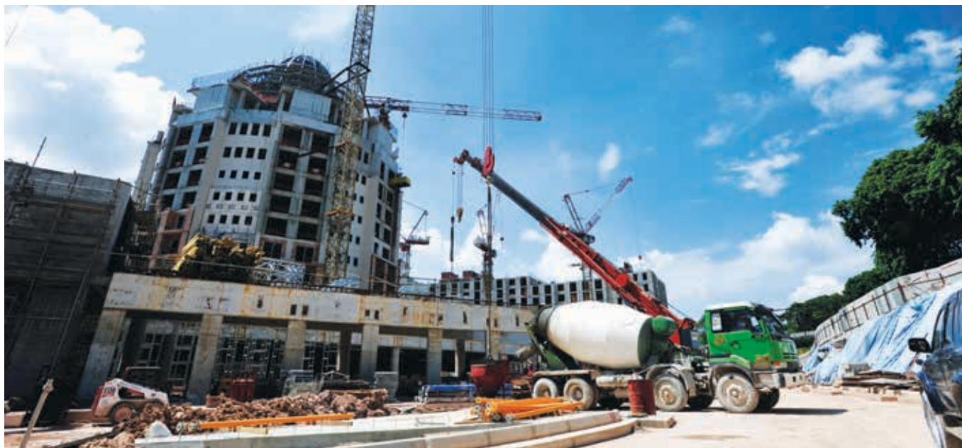
— YTL Cement's blended slag cement using waste aggregates poured for the foundation of Resorts World, Sentosa
