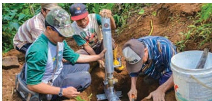
YTLJT's employees providing water access support seen here installing a Hydrant pump system for the community of Kalianan Village
