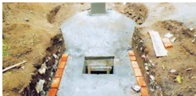
— Construction of a dome-shaped digester engineered to generate biogas from the digestion of cow manure
