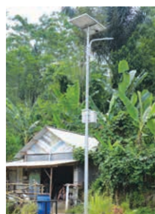
One of the solar lamp units built at Watu Panjang village, as part of the renewable energy programme for rural communities with no access to grid electricity
