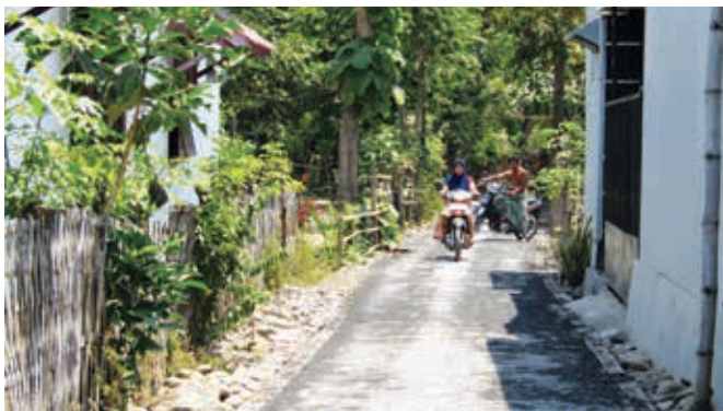
— Roads in rural villages are made with paving blocks produced from fly ash and bottom ash
