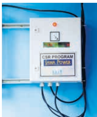
Electricity produced by micro hydro units are regulated by a load controller, designed by YTL Electrical Control and Instrument Team
