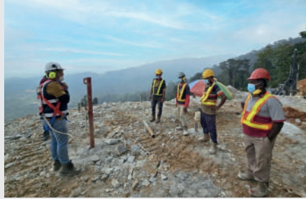
On-site demonstration on the use of fall restraint system at quarry face
