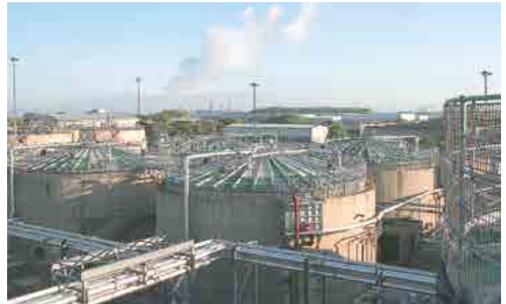
Human waste and food waste collected and processed at GENeco UK's anaerobic digestion facility in Avonmouth, Bristol, UK
