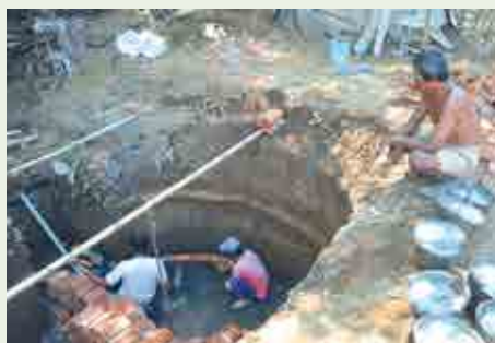
Construction of dome-shaped digesters engineered to generate biogas from the digestion of cow manure
